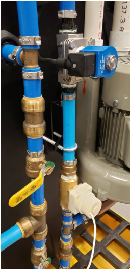
Figure 1 ASV System - Installed
